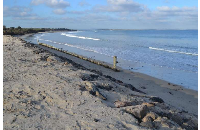
The image shows installation of emergency rock to help protect the Bunurong Road site
